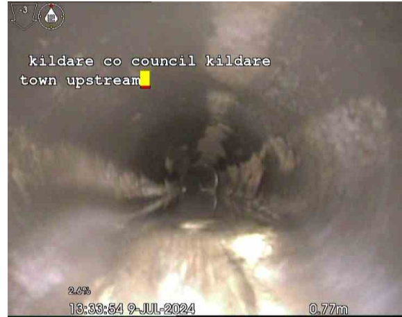
Line AX_c51e83d6-db06-475e-85e5-6e911c16fe16_20240820_17 1919_721.jpg, 00:01:39, 0.00 m Deformed sewer or drain, 10%, Unable to determind distance
