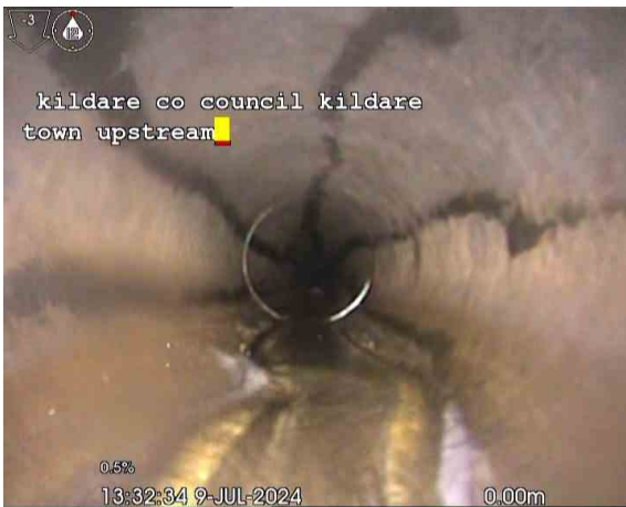
Line AX_ed1b6028-5474-4215-83a9-41bf159f7d4e_20240820_171 844_818.jpg, 00:00:18, 0.00 m Deformed sewer or drain, 10%, Unable to determind distance
