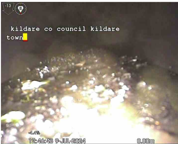
MH 1X_16082024_1451_Sec2_Insp1_SA_0m.jpg, 00:00:13, 0.00 m Survey abandoned, Unable to complete survey due to silt in line
