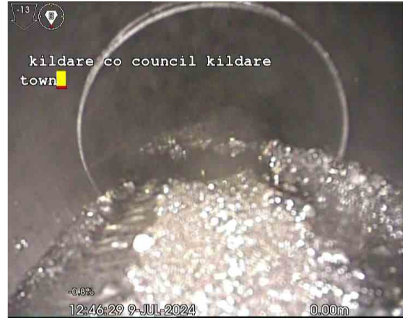
MH 1X_16082024_1451_Sec2_Insp1_DES_0m.jpg, 00:00:00, 0.00 m Settled deposits, fine, 30% cross-sectional area loss
