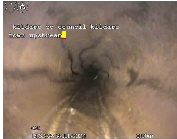
Line AX_20082024_1650_Sec5_Insp1_D_0m.jpg, 00:00:11, 0.00 m Deformed sewer or drain, 5%, Unable to determind distance
