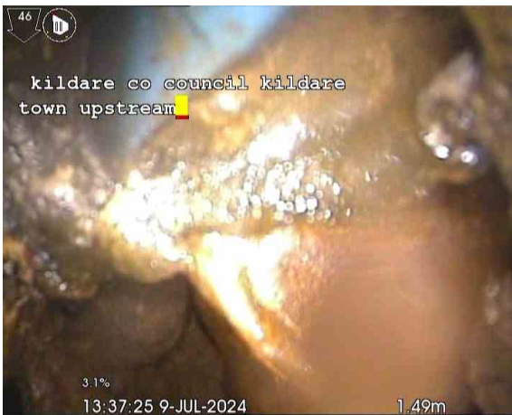
Line AX_20082024_1650_Sec5_Insp1_B_0m.jpg, 00:05:08, 0.00 m Broken pipe from 10 o'clock to 2 o'clock, Unable to determind distance
