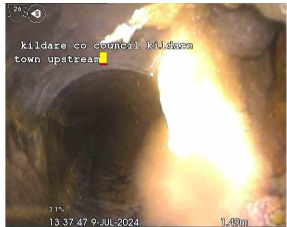
Line AX_20082024_1650_Sec5_Insp1_SA_0m.jpg, 00:05:30, 0.00 m Survey abandoned, Unable to complete survey. Unable to determind distance
