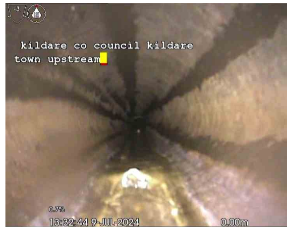
Line AX_6473e9a3-9db9-4550-ad29-d708b40861ce_20240820_17 1854_459.jpg, 00:00:28, 0.00 m Deformed sewer or drain, 10%, Unable to determind distance
