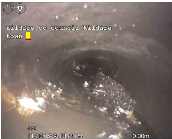
MH 4X_16082024_1451_Sec3_Insp1_SA_0m.jpg, 00:00:15, 0.00 m Survey abandoned, Unable to complete survey due to silt in line
