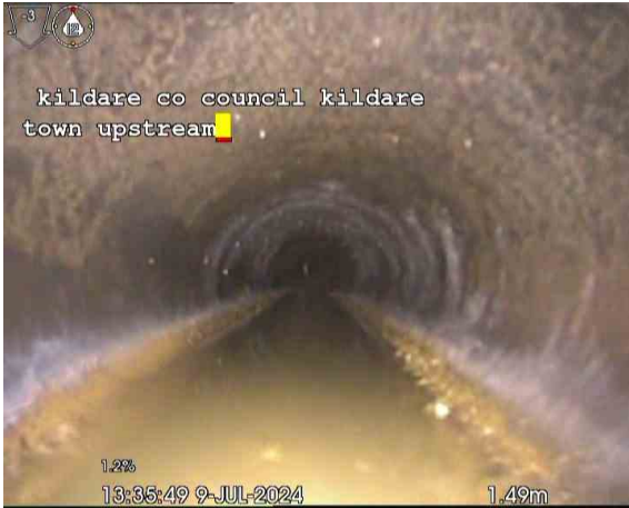
Line AX_cbc976fb-1872-4687-bc74-bfcce0c22b4e_20240820_172 010_969.jpg, 00:03:33, 0.00 m Water level, 15% of the vertical dimension, Unable to determind distance
