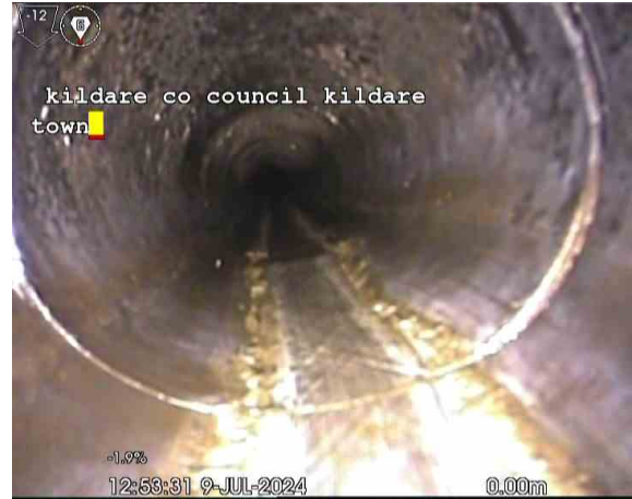
MH 1X_16082024_1451_Sec4_Insp1_SA_0m.jpg, 00:01:28, 0.00 m
